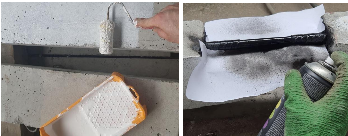
Fig. 2. Application of a white background on concrete (left) and a black background on reinforcement (right)
