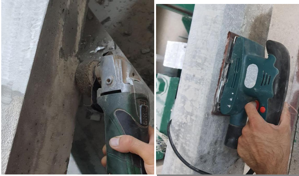
Fig. 1. The process of leveling and cleaning the surface of concrete and reinforcement
